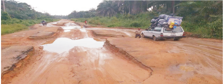
Fig 8: Deplorable state of east west road in south south Nigeria
