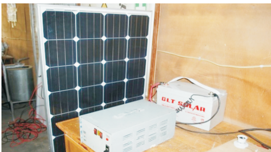
Plate xvi: Inverter and solar panel constructed by 500 level Electrical/Electronics of 2018/2019 academic session.
