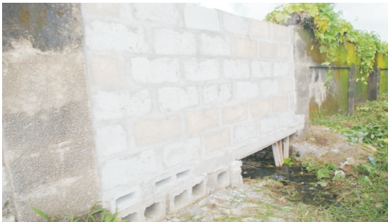
Plate xv: FUT, Minna collapsed fence rebuilt by 500 level Building Technology students of 2018/2019 academic session.
