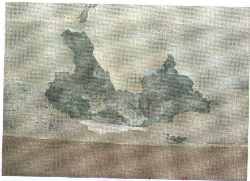
Figure 1: Poor adhesion at paint cement mortar interphase
