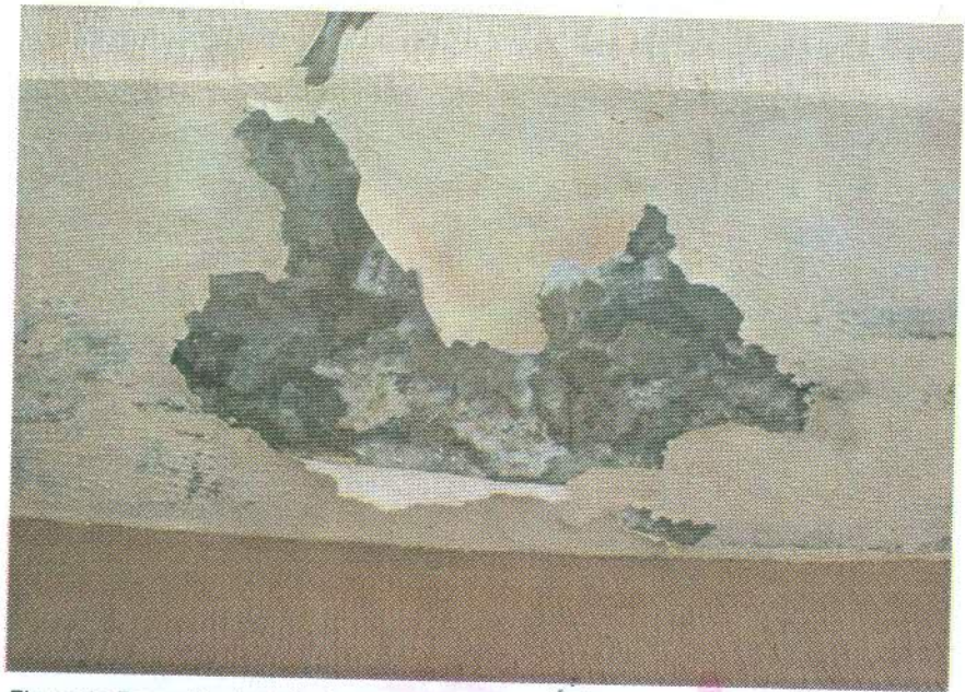
Figure 1: Poor adhesion at paint cement mortar interphase
