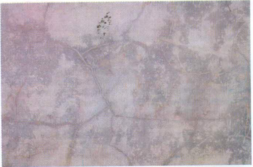
Figure 2: Cracking of sandcrete wall
