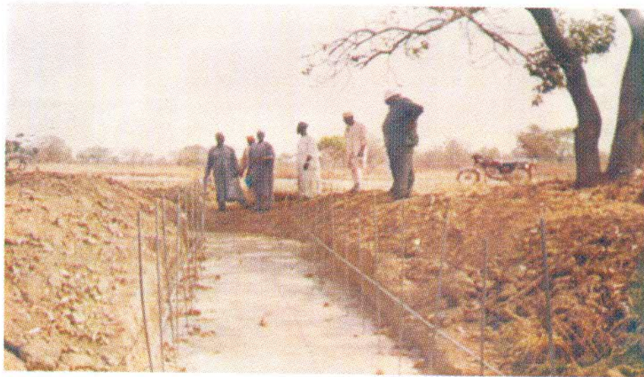
Figure 5: Culvert under construction as part of rural infrastructure development support by Fadama II Project in Lavun Local Government Area of Niger State. (Courtesy of NSFCO, Minna)
