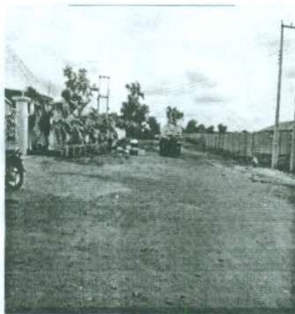
Plate 3.3 - Bad access road
