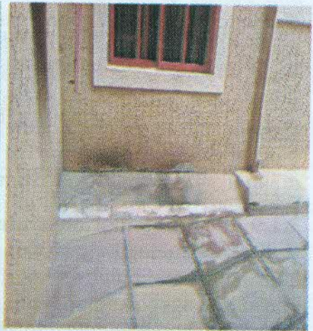
Plate 3.12 - Poor wall and floor maintenance
