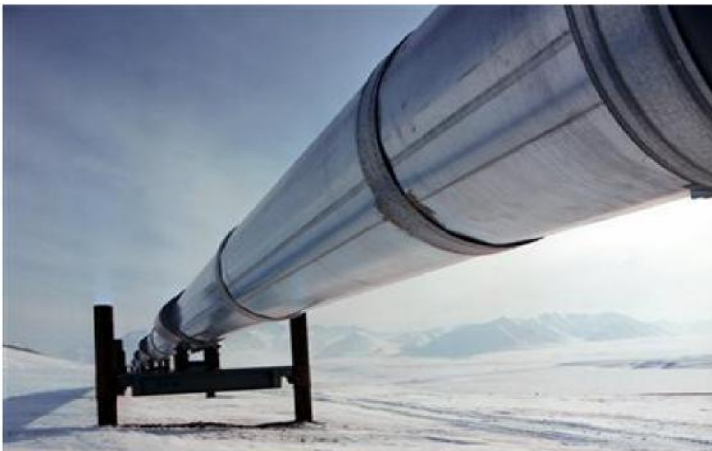
Figure 20: Natural Gas Pipeline (Nasir et al, 2012)
