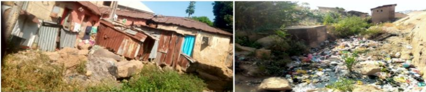
Plate III: The state of the buildings and the environment of informal settlements in Jenta-Adamu area, Jos, Plateau State (Source: Researchers' field survey, 2021).
