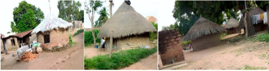
Plate I: Unauthorised building subdivision, building materials and building conditions in Gaadi area, Makurdi, Benue State (Source: Researchers' field survey, 2021)
