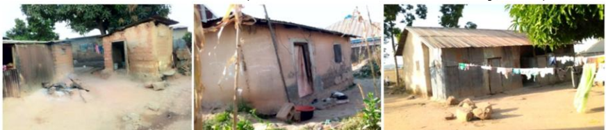
Plate V: Building condition of kitchen and dwellings in informal settlements of Utan area, Jos, Plateau State (Source: Researchers' field survey, 2021).
